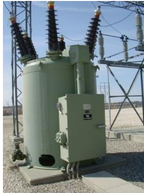
Gambar 6.13. Oil Circuit Breaker
